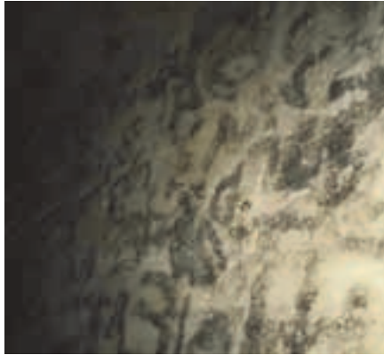
The Apotropaic 'Sooty Graffiti' on original 17C plaster Eave at Ferriers
